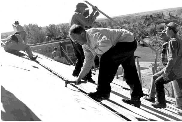
Parishioners roofing St. Patrick's in their spare time, some still in their office attire!
